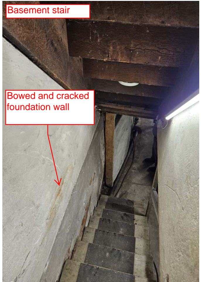
Bowed and cracked foundation wall
