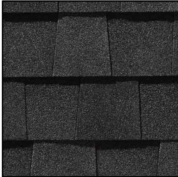
ROOF SHINGLES: CERTAINTEED "LIFESTYLE SERIES" DESIGNER ASPHALT ROOF SHINGLES COLOR = "MOIRE BLACK"
