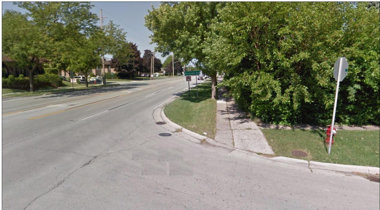
Figure G1 - Current conditions of sidepath (retrofitted from sidewalk) along Central, at Walnut. Although along the framework route, it is not appropriate as a bikeway, due to pavement condition and encroachment of vegetation.
